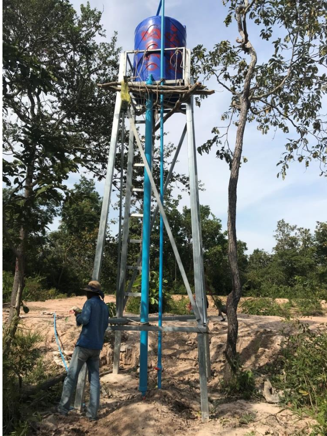
Figure 14. Water tank installed
